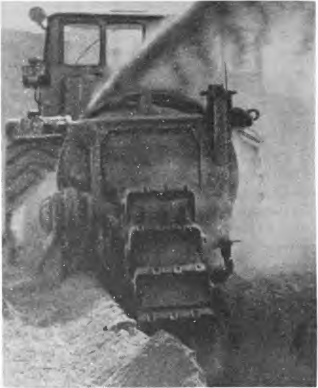
Figure 6-54. Ditching machine. Engineers use specialized machinery such as this automatic ditching machine, along with bulldozers, cranes, and other heavy equipment.
